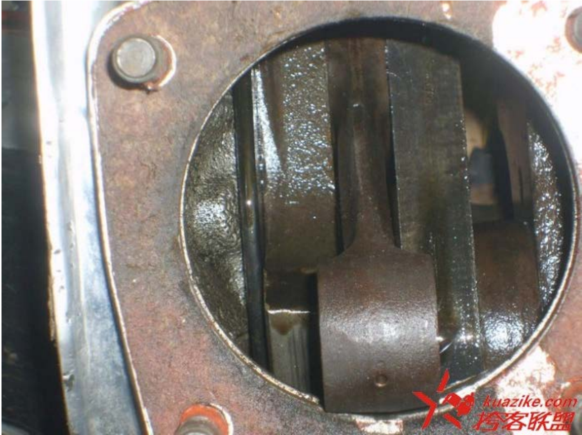
这是前挡油盘照片，间隙正常。This photo is of the front oil slinger, showing normal clearance.
